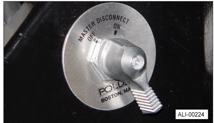
Cut-Off Switch Mounted in Cab of Truck.
